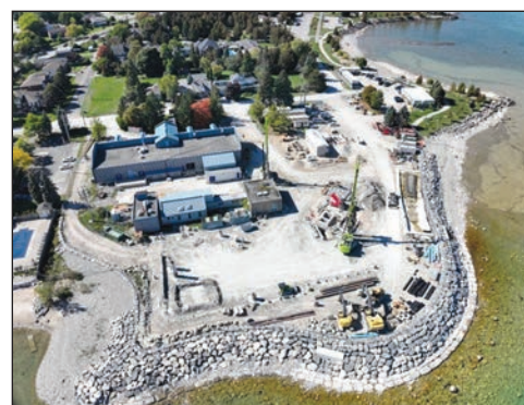
AERIAL SHOT – The Raymond A. Baker Water Treatment Plant, from an aerial view, shows ongoing construction for its expansion. CONTRIBUTED PHOTO
